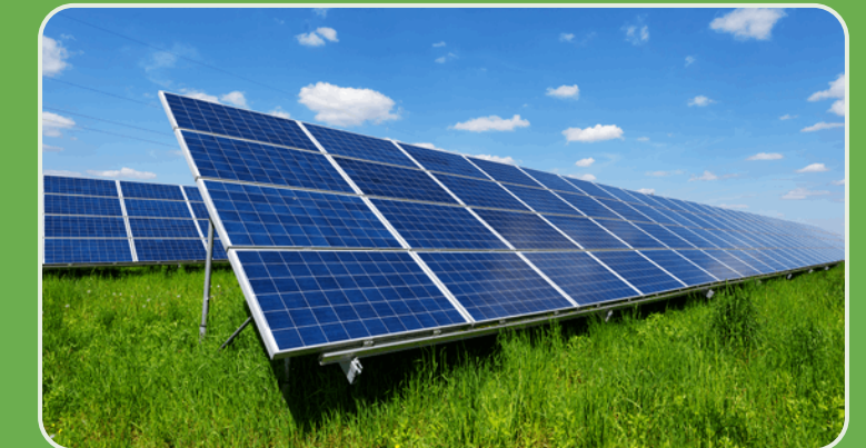
WORLD'S LARGEST SOLAR PARK 5000 MW
