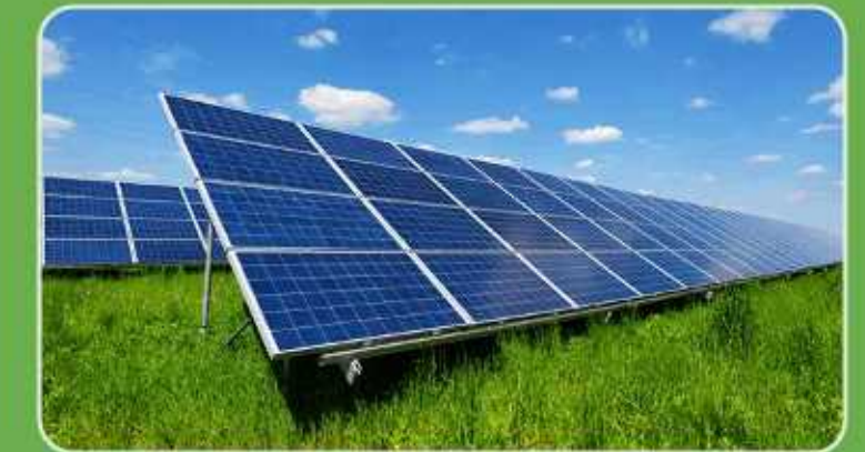
WORLD'S LARGEST SOLAR PARK 5000 MW
